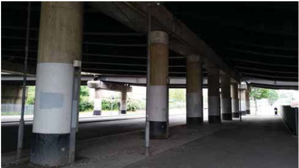
Photo: Pigeon defecation on footpaths under bridges, as seen here under the M5 at Oldbury.
